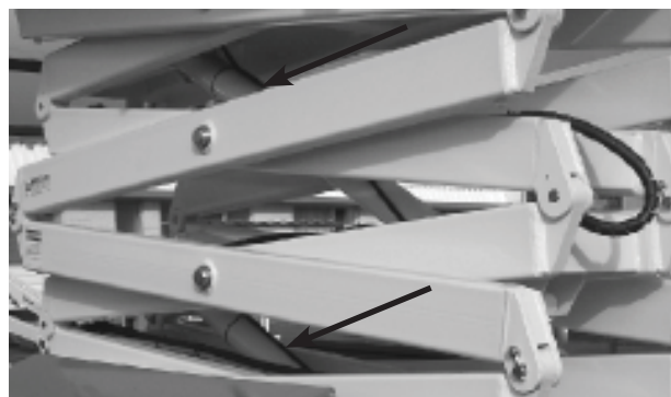
Figure 7.15 - Check Hydraulic Cylinders
