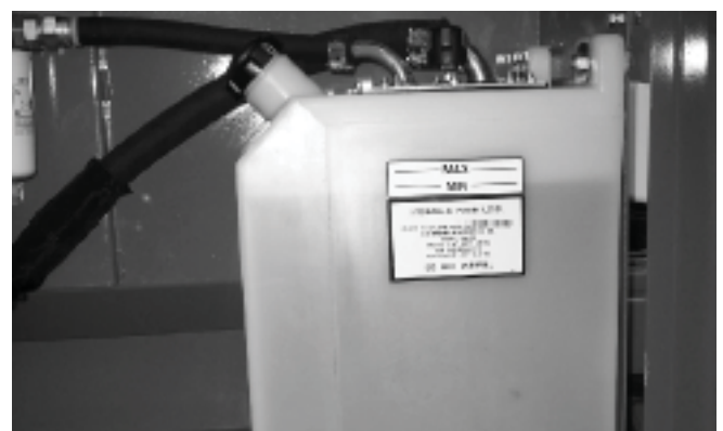
Figure 4.4 - Hydraulic Oil Level
