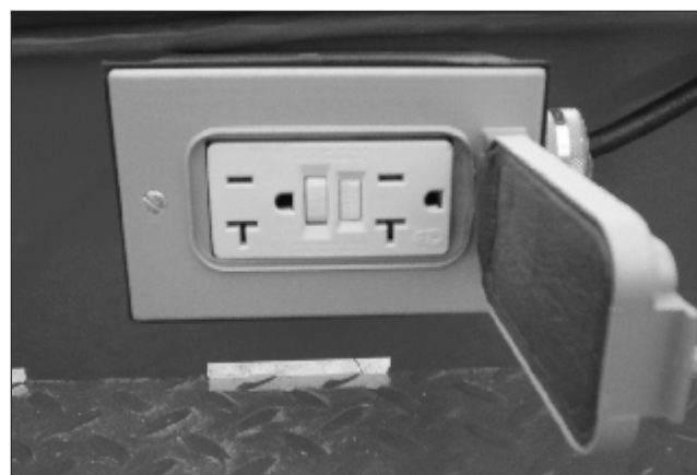
Figure 9.8 – Electrical Power Outlet
