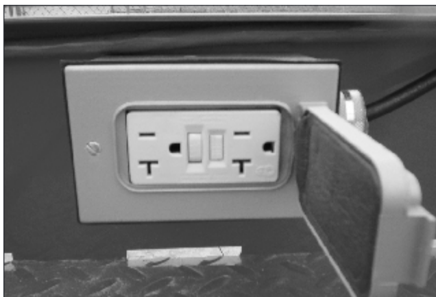
Figure 4.7 – Electrical Power Outlet
